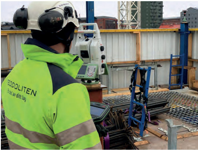
▲ A total station operator sighting the four active GNSS control points to determine the coordinates of the instrument and the orientation of the primary axis.
